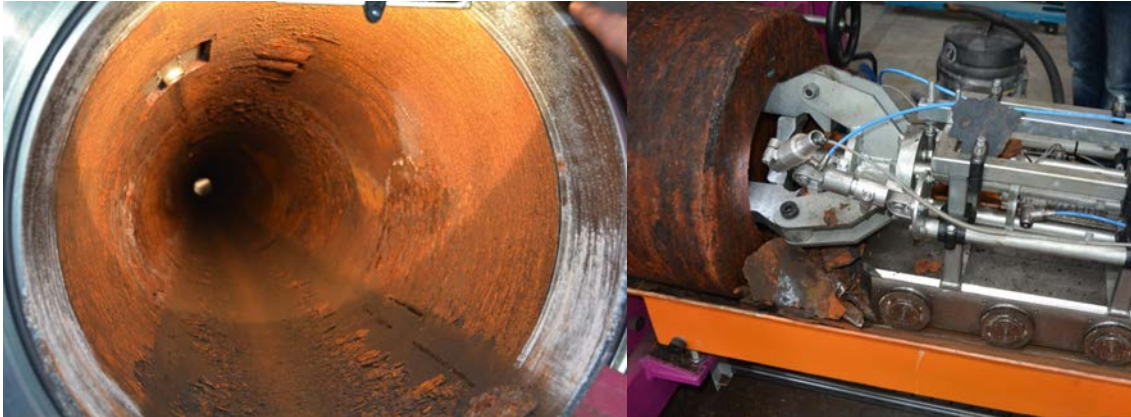
Figure 6 – Rust production inside the liner (left) and build-up at package contact (right)
