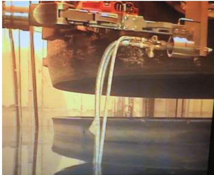
Fig. 6. Cut of the RPV, in the foreground the burner Retaining the rotation and the cutting parameters a horizontal full circle had been cut within 120 min and without interruptions. Subsequent the manipulator with the burner was slewed away and the flange and nozzle area of the cylindrical part of the RPV was lifted (see Fig. 6) and transported to the cutting area room 01.412 (see Fig. 7)
