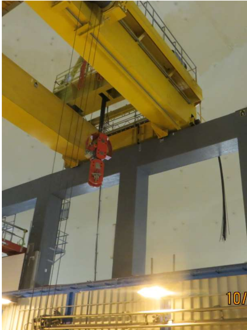
Fig. 3. Strand jack with connection block on the bridge of the reactor building crane
