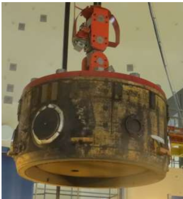
Fig. 7. Transport of the RPV flange and nozzle area to the cutting area room
