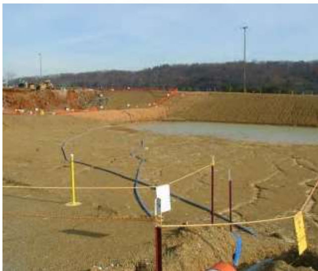
FIGURE 7. EMWMF WASTE CELL 2 FLOODING [8].
