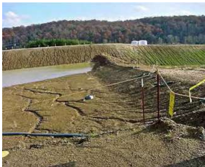
FIGURE 8. EMWMF REPAIRED CELL BERM [8].
