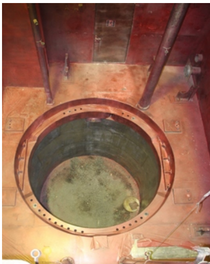
Fig.4. Final condition of the MR reactor pool after dismantle of intra case elements
