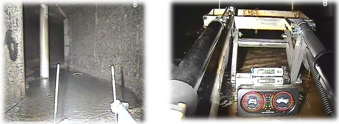
Fig. 17 a&b. Water Hazard inside Exhaust
