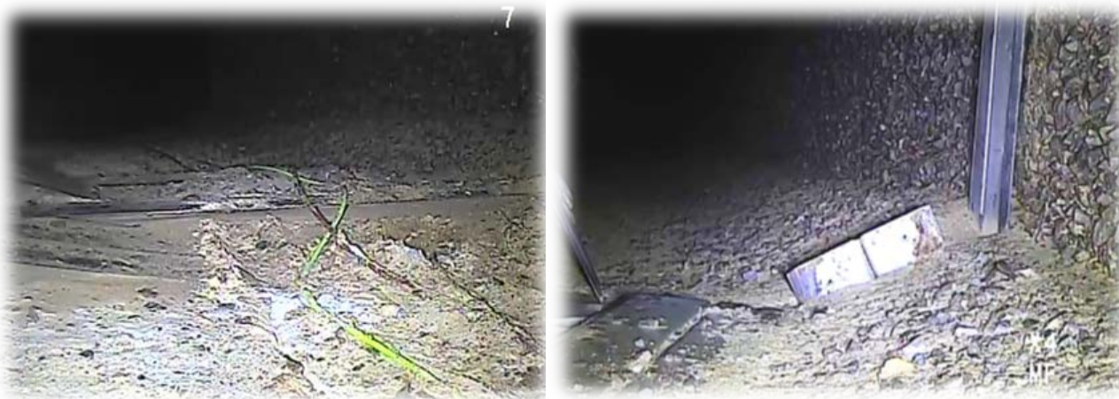
Fig. 19 a&b. Expansion Joint Debris inside Exhaust Tunnel
