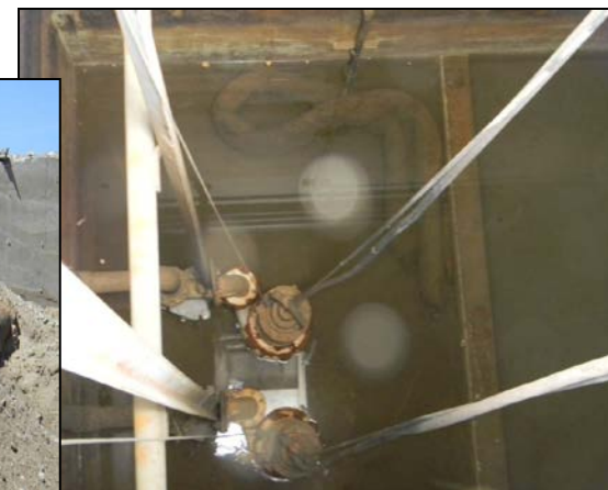
Collection Sump, April 2014
