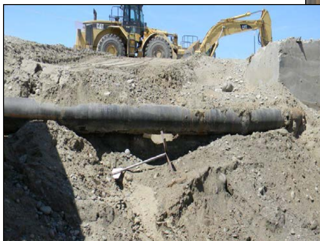
Process sewer inlet piping , July 30, 2014
