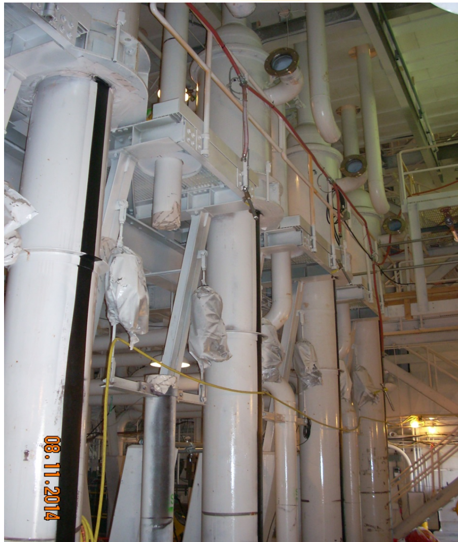
Four of the nine heat exchangers to be treated in MFC-767
