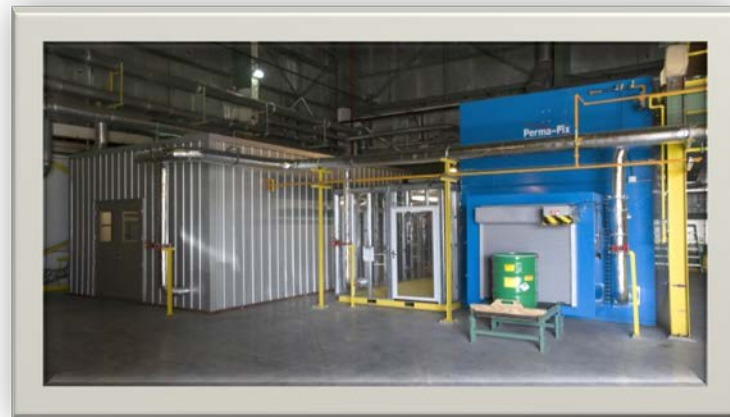
Tritium Processing Enclosure
