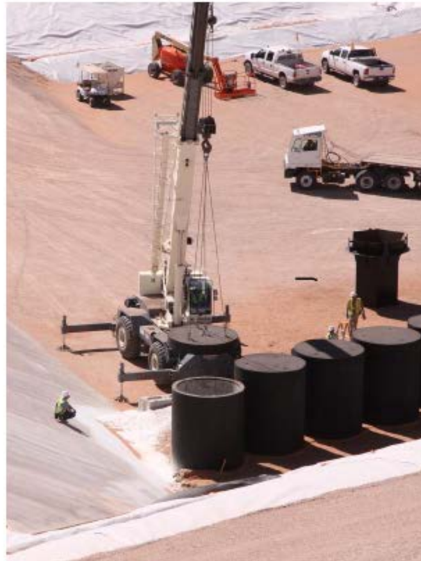
MCC Opened for Waste Placement
