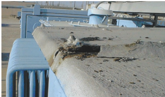
H-Area Switch Gear Roof
