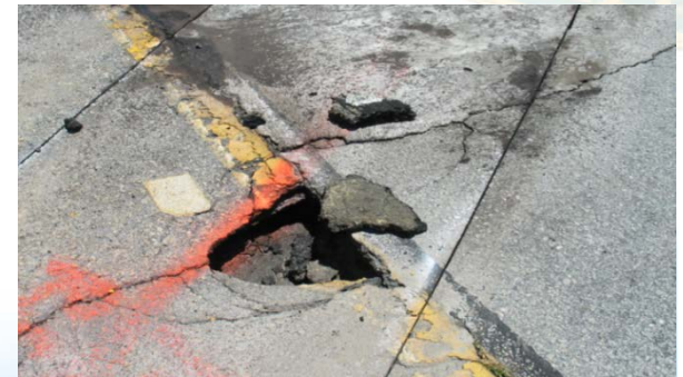
C-Road Drain Failure
