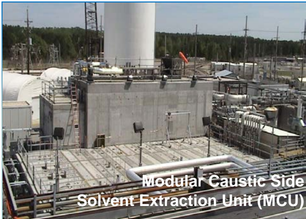
Centrifugal Contactor Bank
