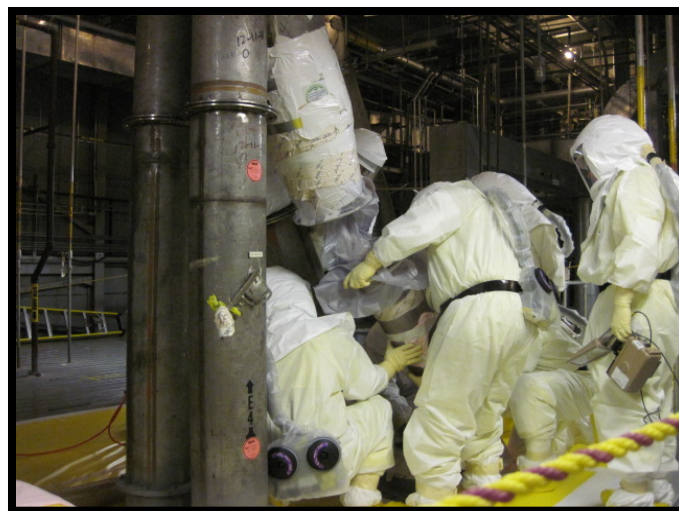
Employees in the duct level separate, bag and remove sections of E4 ventilation duct.
