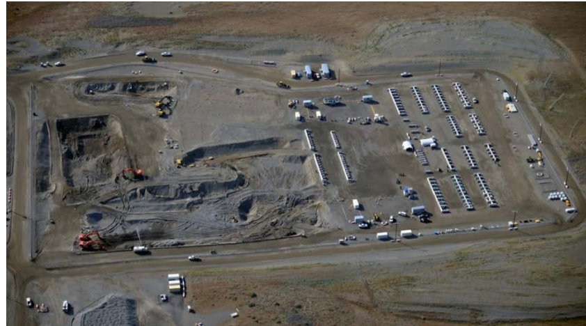
The 618-10 Burial Ground is one of the most highly contaminated waste sites on the River Corridor.
