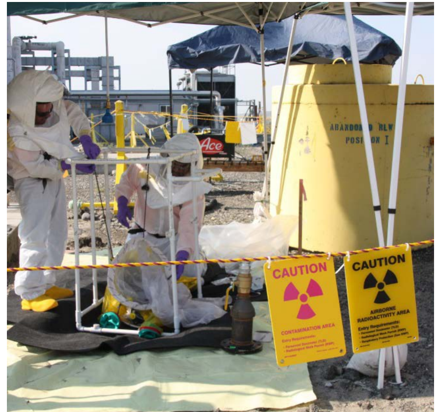
Radiological Liquid Waste System piping in the 300 Area was stabilized, removed, and disposed of at ERDF.
