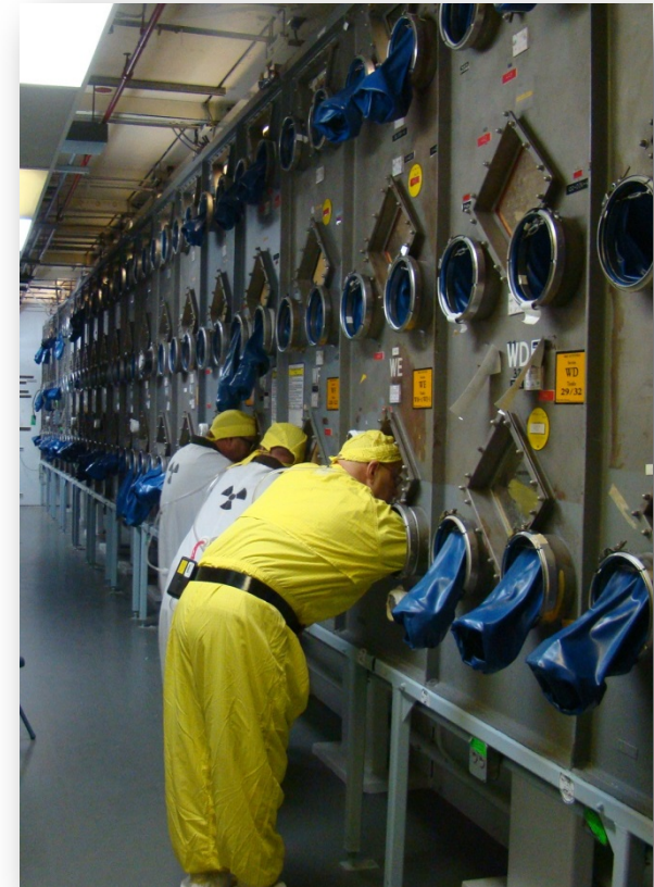
One of two column glove boxes that will be prepared to remove during demolition
