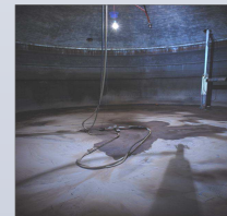
Figure 5. SRS Tank 19 After Cleaning
