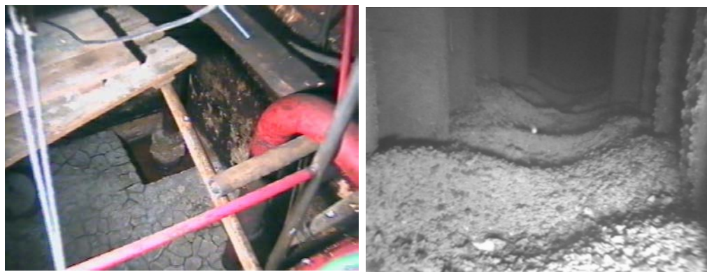
Fig. 4. Presence of the sludge on the bottom of different tanks
