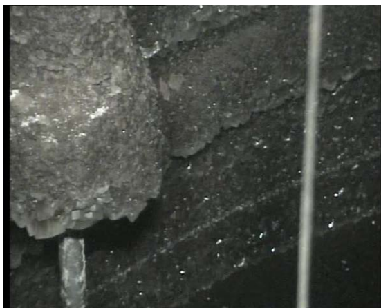
Fig. 7. Crystalline sediments on the walls of the tank N. ZT10N-8
