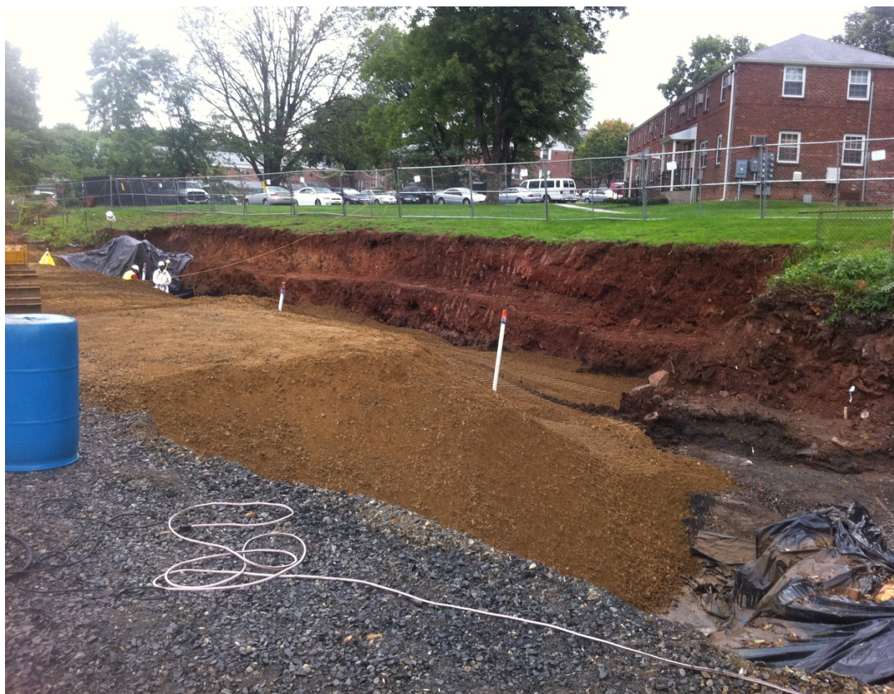
Fig. 3. Garden apartments community viewed from the 111 Essex Street vicinity property. The white stakes approximate the property line. Coles Brook is not shown as it was diverted to a pipe at the time of this photo.
