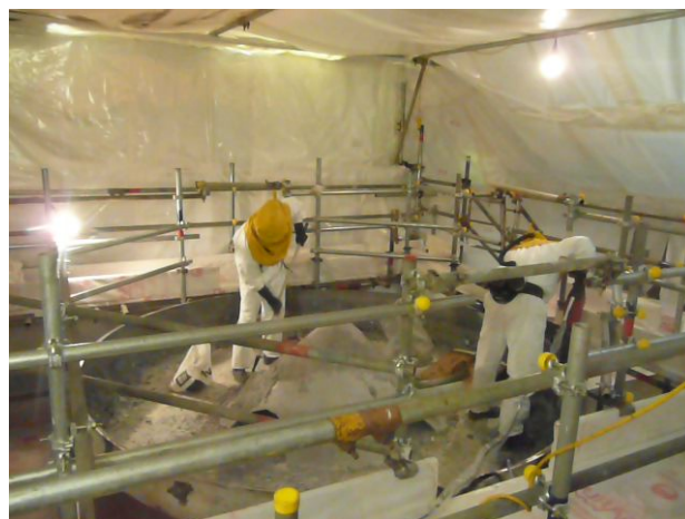
Figure 12: Workers Removing the Sodium from the Bottom Dome in the Temporary Processing Tent
