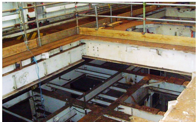
Figure 6: Example of a Layer of Structural Steel Requiring Removal to Access a Tank
