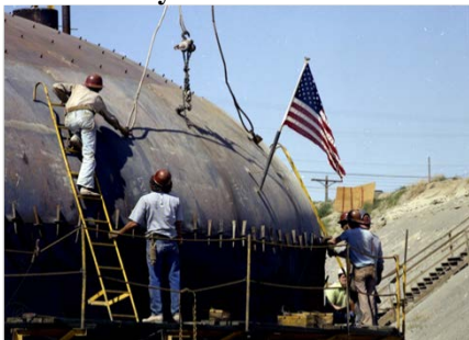
Secondary Liner Top Knuckle
