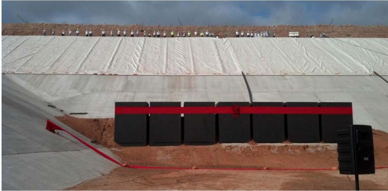
Photo No. 1 – WCS Federal Facility with rectangular MCCs in the background ready to be loaded.
