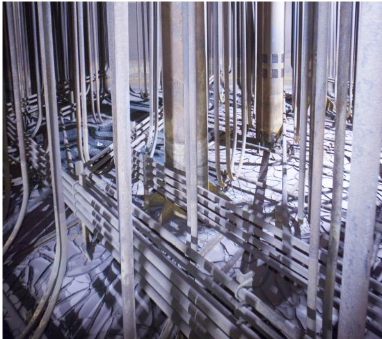
Figure 3 - Tank 5F Cooling Coil Obstructions
