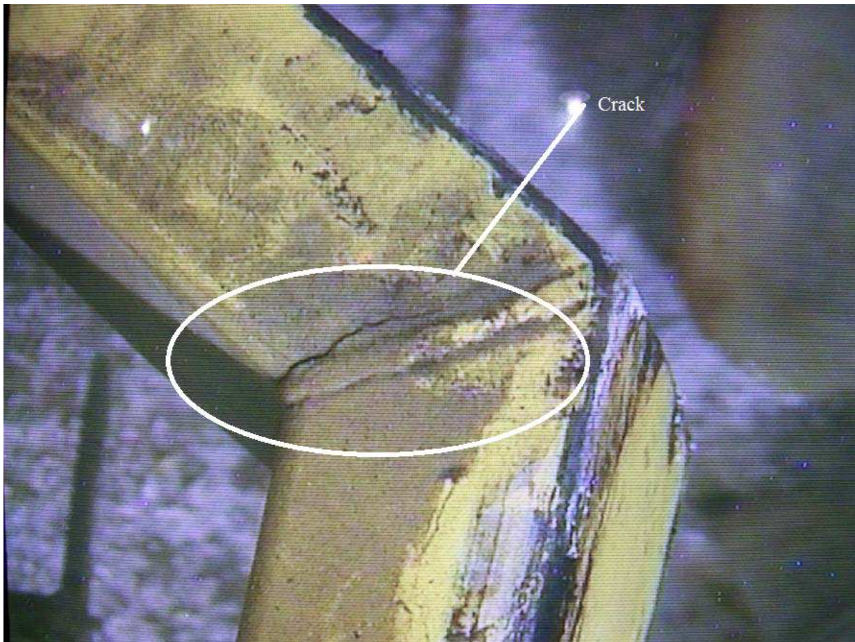
Fig. 4 Upper arm weldment crack
