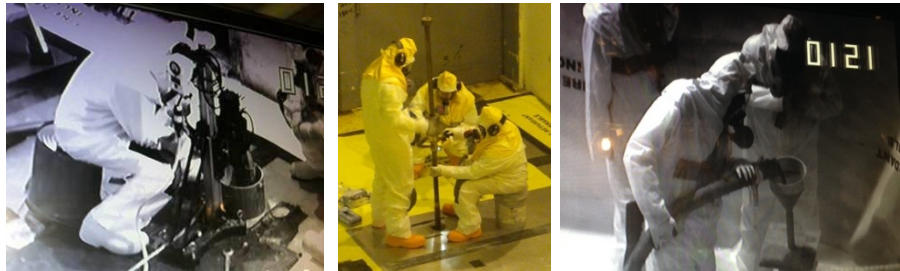
Fig. 12, Fig. 13, Fig. 14 and Fig. 15. Draining pit, core boring, subsurface soil testing, and grouting the void spaces in a high contamination and radiation area.
