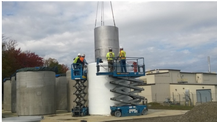
Fig. 3. Overpack being loaded into a cask
