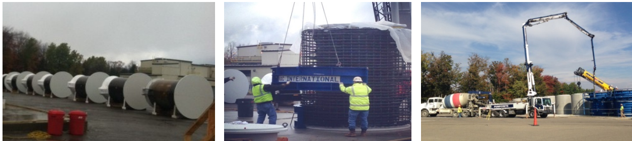
Fig. 1. Cask liners delivered, fitted with rebar, and concrete placed to form the West Valley casks. Canister Overpack
