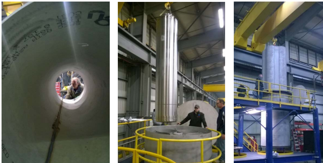
Fig. 2. Basket cell inspection, lowering canister into basket, and lowering basket into Overpack.
