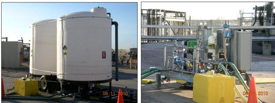
Figure 7. DWS System: Two 11 m 3 tanks (left) and PLC with valves and instrumentation (right)
