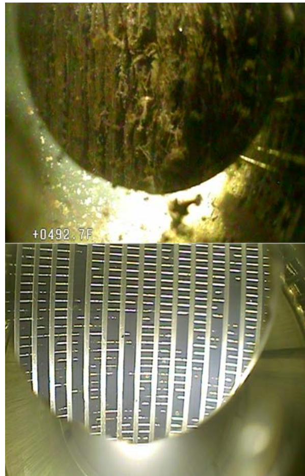
Fig. 1. Injection well screen before rehabilitation and after one rehabilitation in October 2013. Note the clogging metal oxides remaining on the well screen after rehabilitation.
