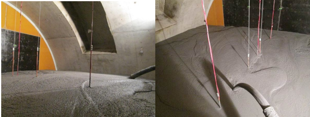
Fig. 6 – Easy pouring and even emplacement of low pH SCC inside the test box
