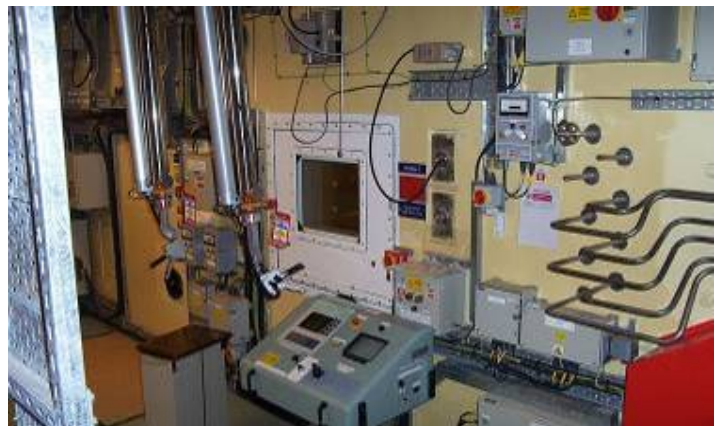
Figure 4 – Typical operator control console and MSM arrangement.
