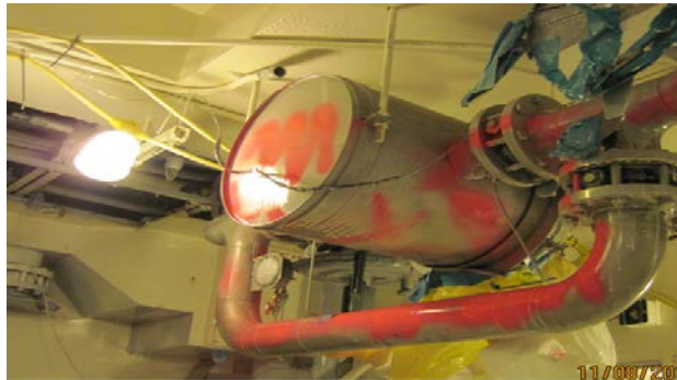
Figure 2: Brightly colored spray painted identified contaminated items that were left in place during demolition of the 209E Critical Mass Laboratory at Hanford in 2011. That facility contained plutonium-bearing source term and was demolished safely and compliantly.
