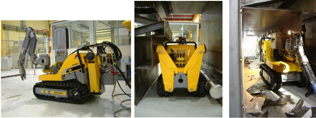
Figure 7: a) Brokk 90 equipped with an on-board controller and the Cybernétix Maestro arm; b) the machine in the technical gallery mock-up; c) in action with a nibbler.
