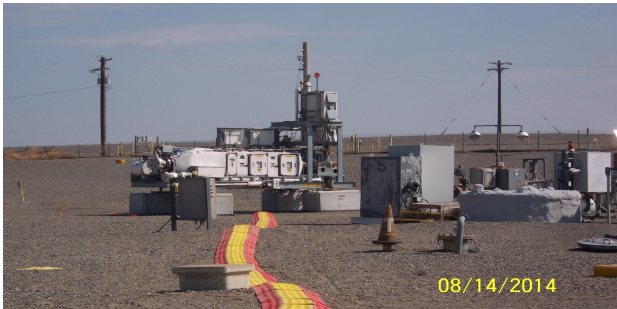
Figure 2. Portable Exhauster Skid in 241-T Tank Farm.
