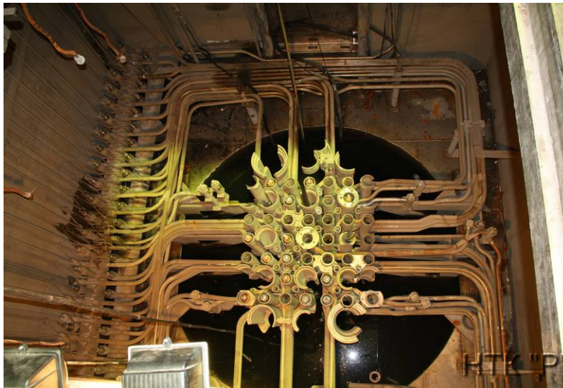
Fig. 3 Upper tie plate and upper core basket of reactor MR.
