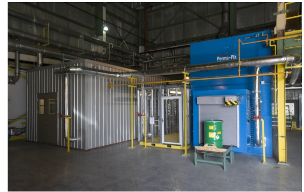
Tritium Treatment Enclosure
