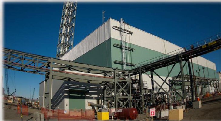
Overhead pipe racks for steam and glass formers
