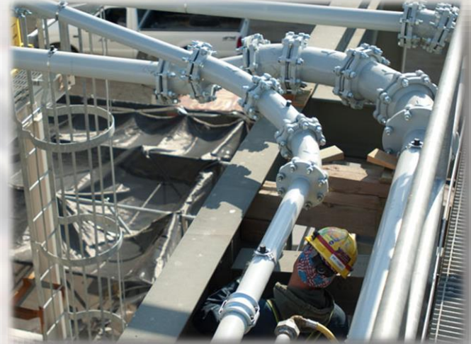
Glass former piping
