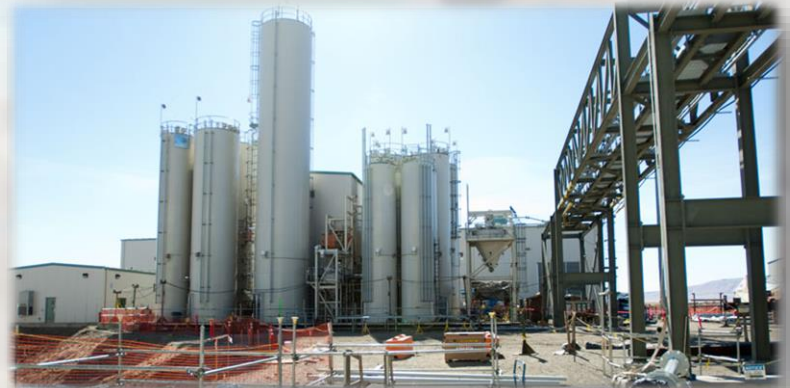
Glass former silos
