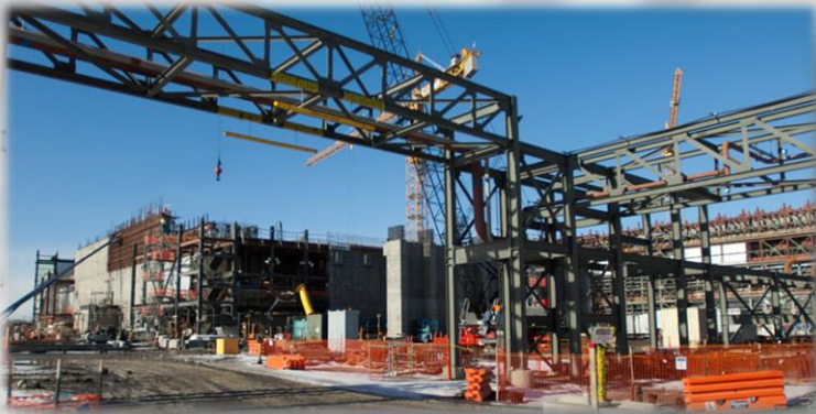
Overhead pipe racks for steam and glass former materials
