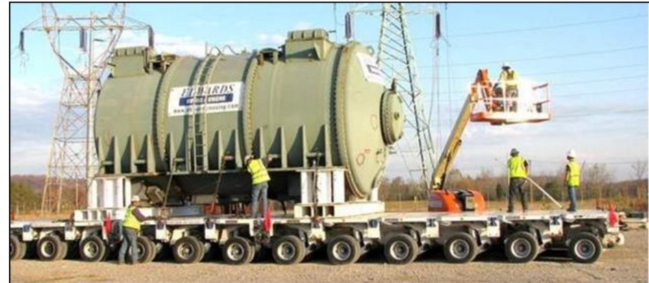
200-ton synchronous condenser
