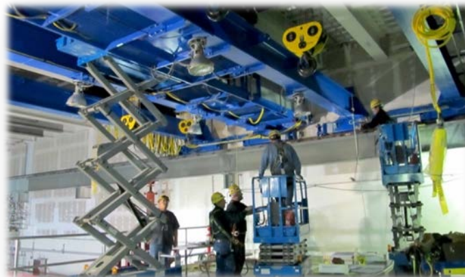
A 25-ton crane is being installed to continue work on the Low-Activity Waste Facility melters
