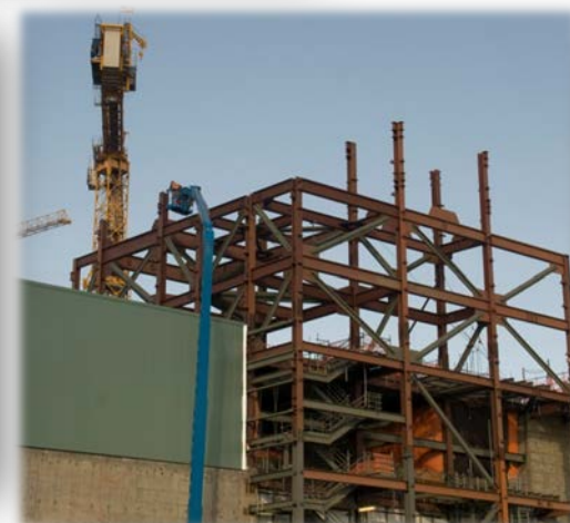
Employees continue installing structural steel at the 77-foot elevation of the High-Level Waste Facility
