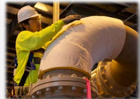
An employee covers pipe with insulation in the Balance of Facilities chiller compressor plant
