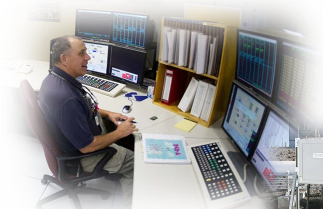
242-A Evaporator control room
