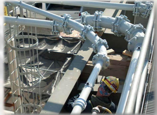
Glass former piping
