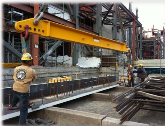
Ironworkers begin rigging a steel beam to be lifted into the High-Level Waste Facility
