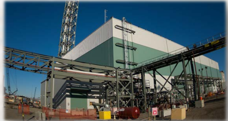
Overhead pipe racks for steam and glass formers
