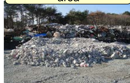
Unit 5 / 6 north side storage area
