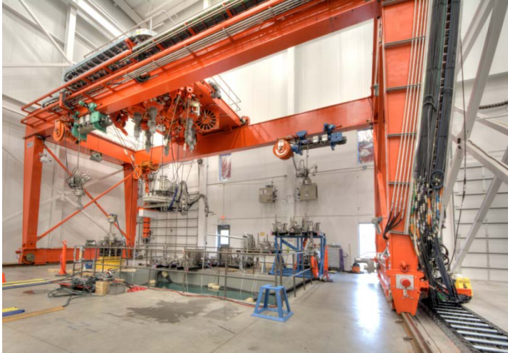
Figure 1: Fukushima 1F-3 Spent Fuel Removal System
