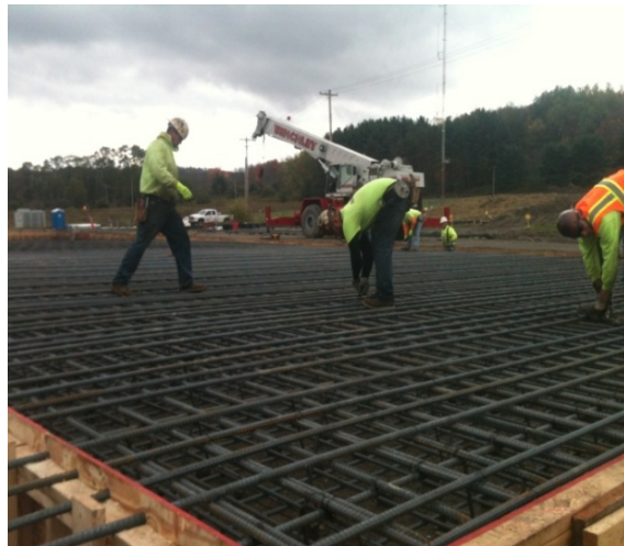
Picture 5 A total of 243 tons of rebar was installed for the storage pad and apron.
