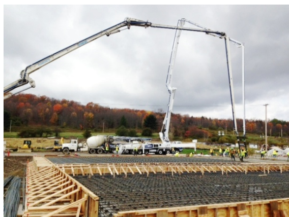
Picture 6 Construction of the main storage pad required approximately 1,800 cubic yards of concrete.
