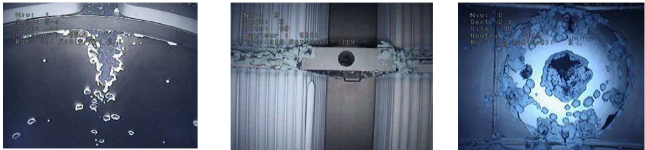
Fig. 4. Corrosion of the Ni plated metal surfaces
