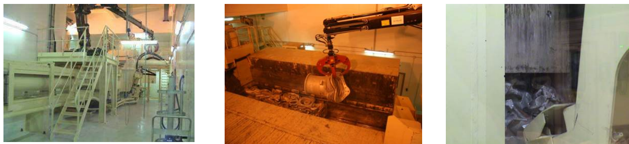
Fig. 8. The super compactor used for the dismantling of the UDG military plant
