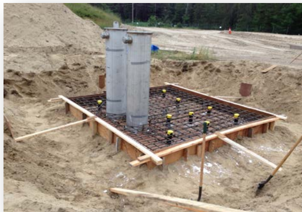
Fig.3 The installed risers and rebar on ALWT-1 prior to the concrete pour to provide adequate reinforcing of the tank lid.
