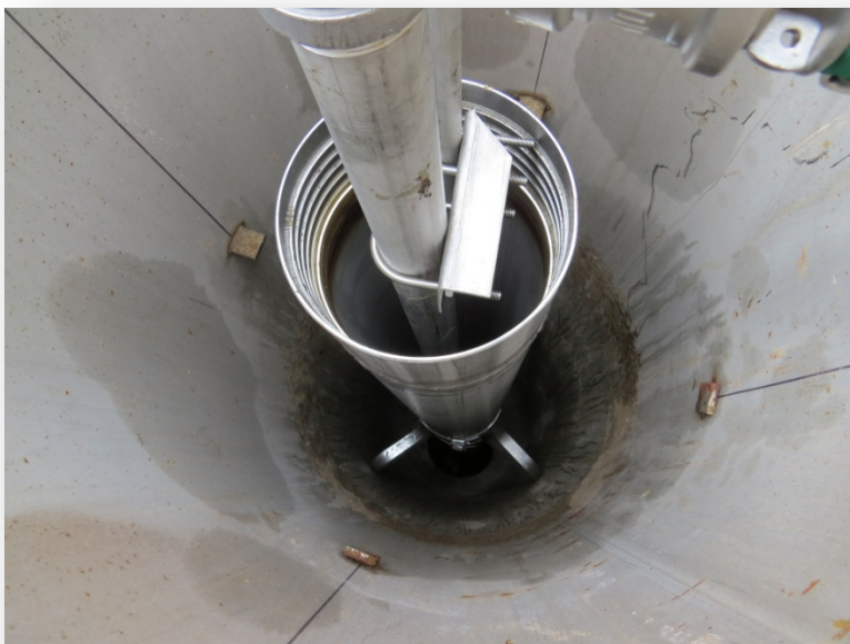
Fig.4. A view down the riser of ALWT-2 showing the extraction pipes installed within the standpipe.
