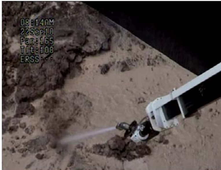
Figure 8 - Prototype ERSS Testing at the Hanford Cold Test Facility
