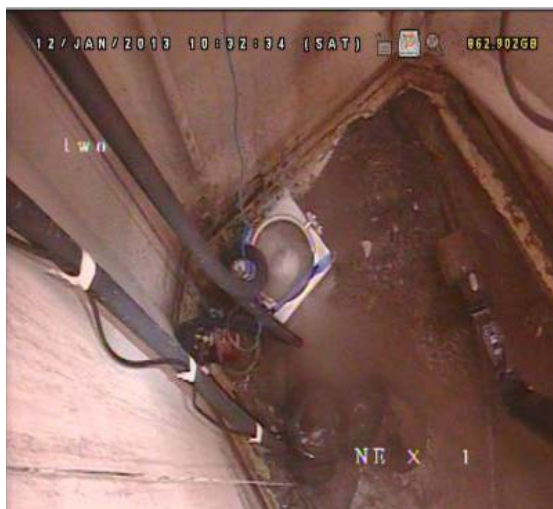
Fig 6. Wash station installed in PNV.
