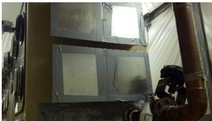
Figure 2: Ventilation ports after plenum removal
