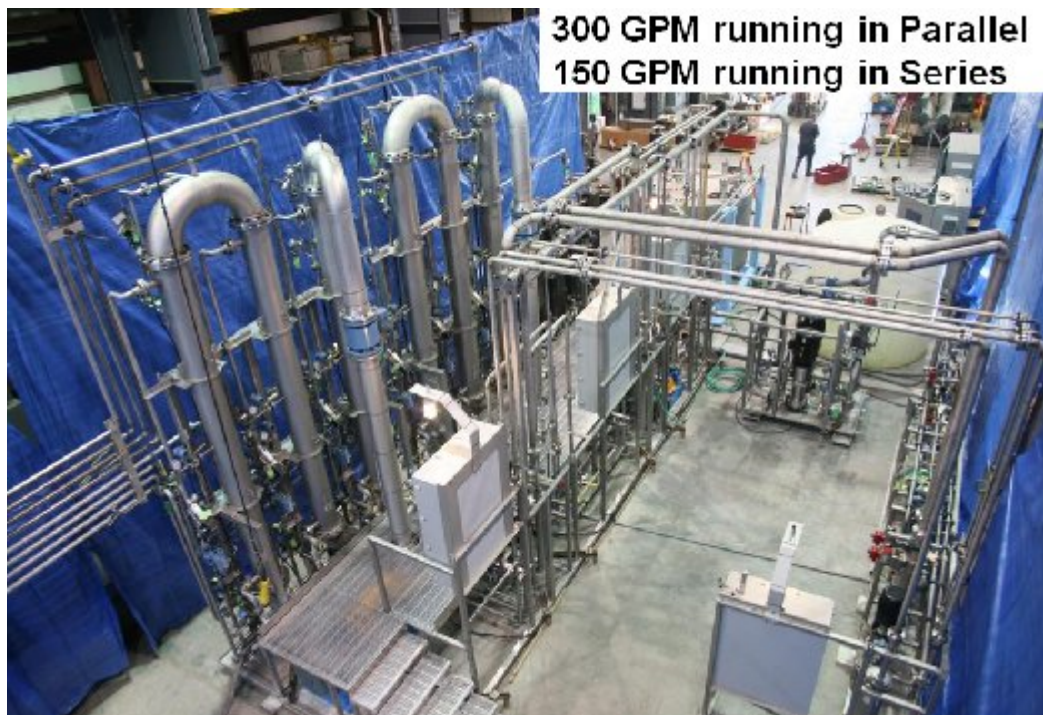
Figure 6 - Picture of the full size system after construction
