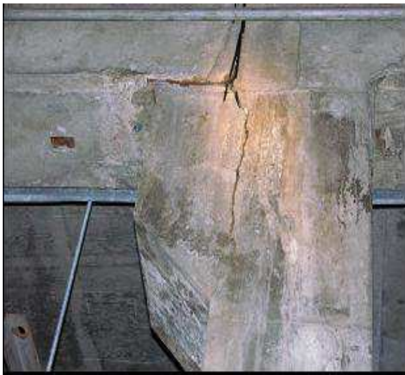
Figure 1. Structural failure of a corbel could have caused a catastrophic failure of the floor system.
