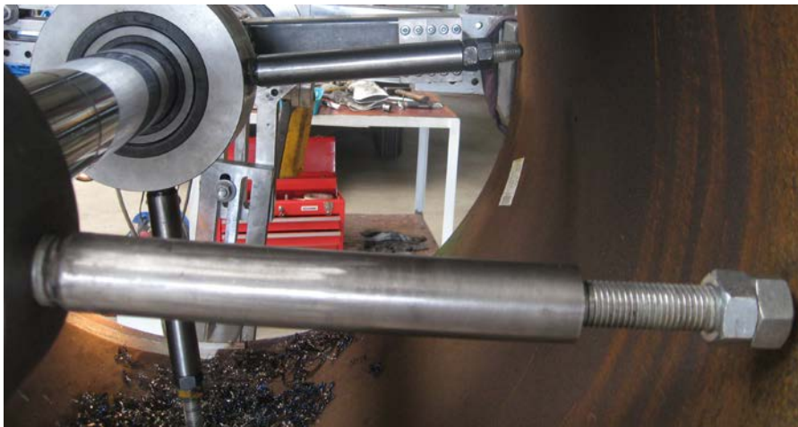
Figure 3: pipe from inside
