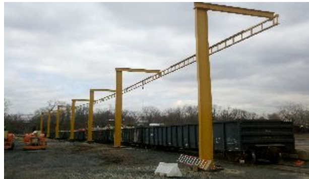
Figure 4 – Rigid Fall Arrest System at Maywood, NJ
