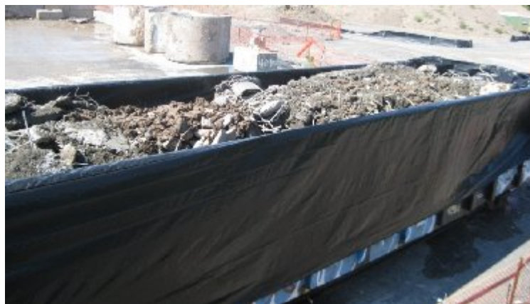
Figure 8: Strain and sprain, cut, and impalement hazards visible prior to liner closure.
