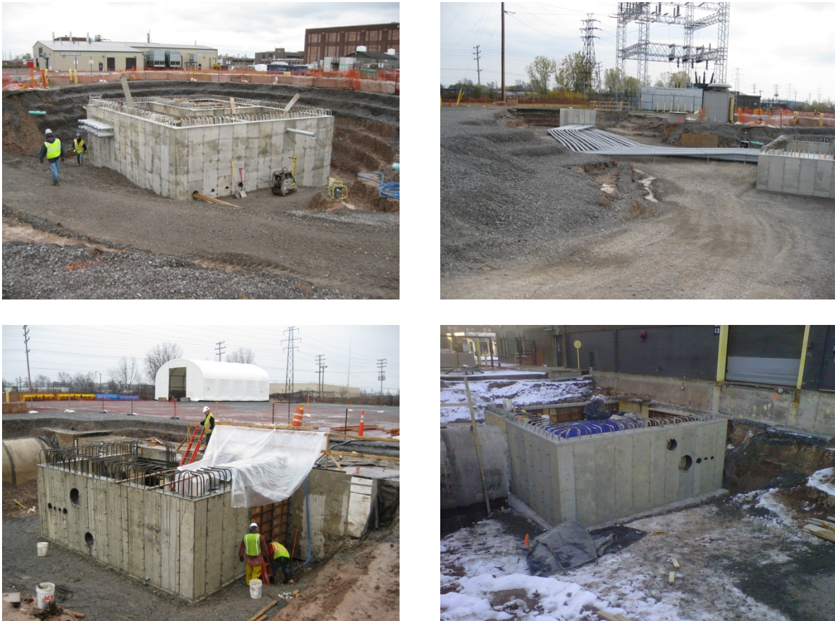
Fig. 6. From top left to bottom right, JB 7A, electrical vault (with extension) and conduits for duct bank, JB 8A, and JB 9A.
