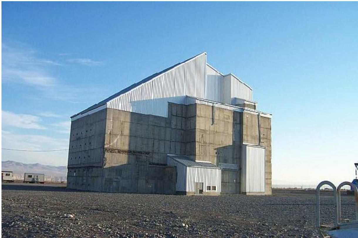
Fig. 4. D Reactor SSE beginning to show change to sloped shed roof design
