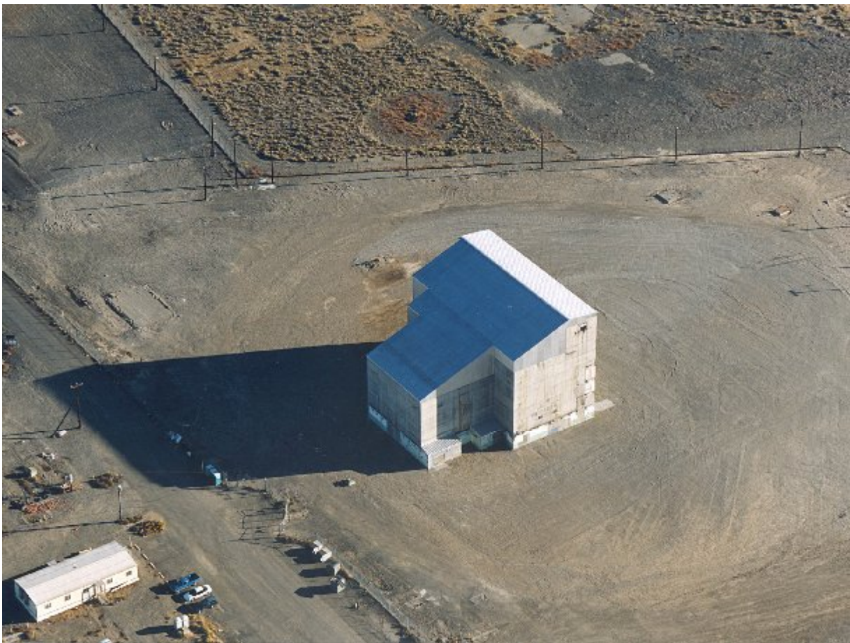
Fig. 1. C Reactor SSE shows low roof slope from removal of all existing roof structures above concrete.
