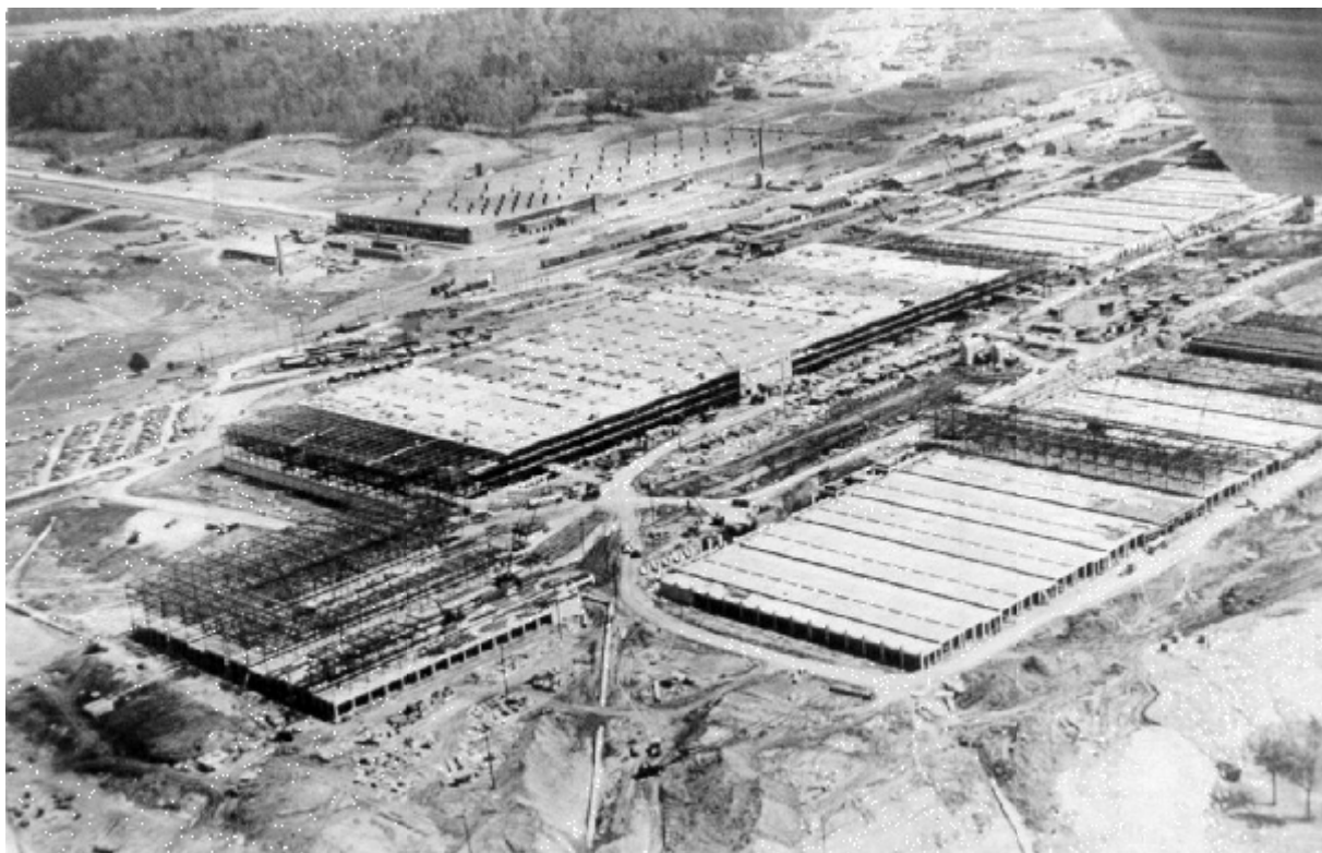
Figure 1. View during construction of the enormous U-shaped K-25 Building, looking Southeast - April, 1944
