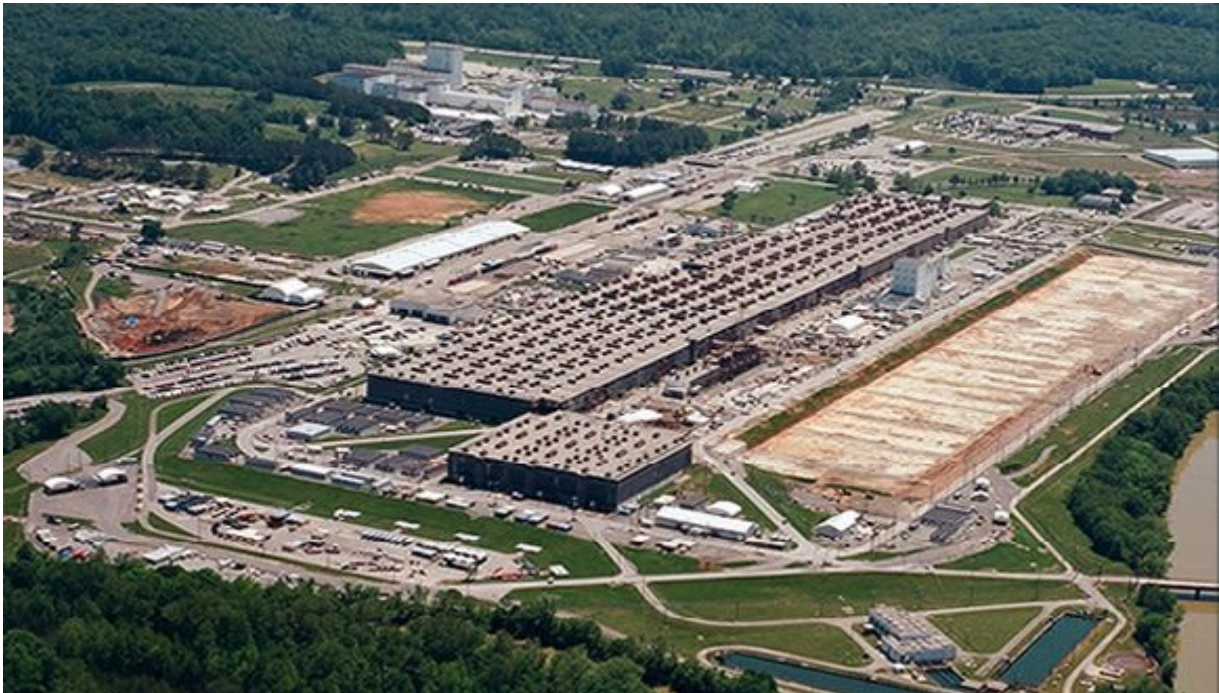
Figure 2. View during demolition of the enormous U-shaped K-25 Building, looking Southeast - July, 2012
