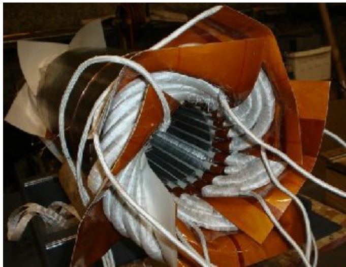
Figure 5 – Transfer Pump Stator Electrical Winding
